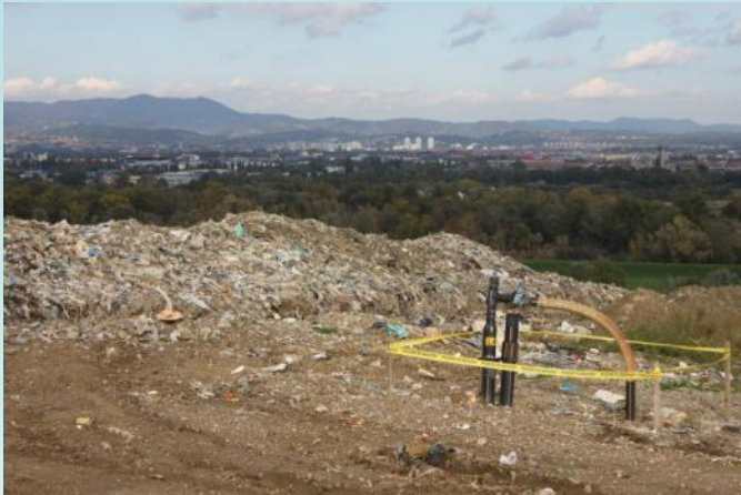
Gas recovery of landfill site (Zagreb, Croatia)
