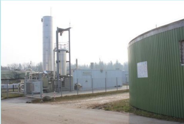
Upgrading unit (Bavaria)
